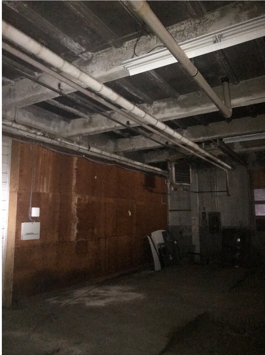
Photograph – 2: Photo depicts the typical condition of asbestos thermal pipe insulation throughout the structure located at 32-60 Ernest Street; Providence, RI.
