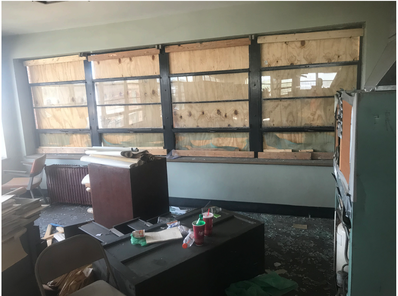
Photograph – 4: Photo depicts the typical condition and application of asbestos vinyl flooring, vinyl cove molding and AMC/PACM window system within the structure located at 32-60 Ernest Street; Providence, RI.
