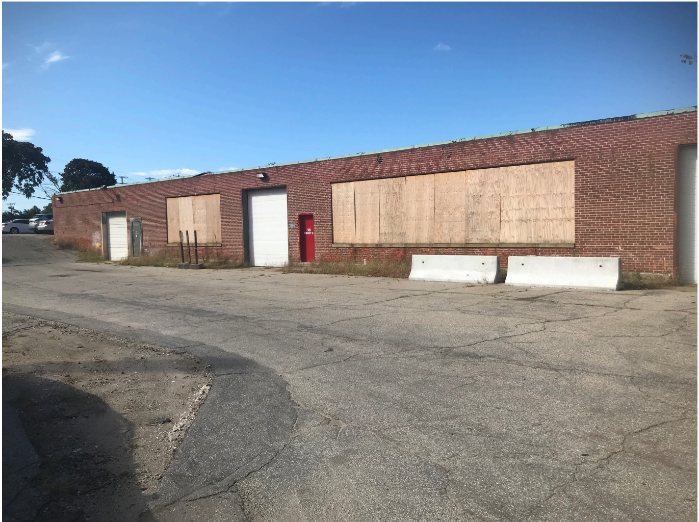
Photograph – 1: Photo depicts the typical condition of the structure as located at 32-60 Ernest Street; Providence, RI.
