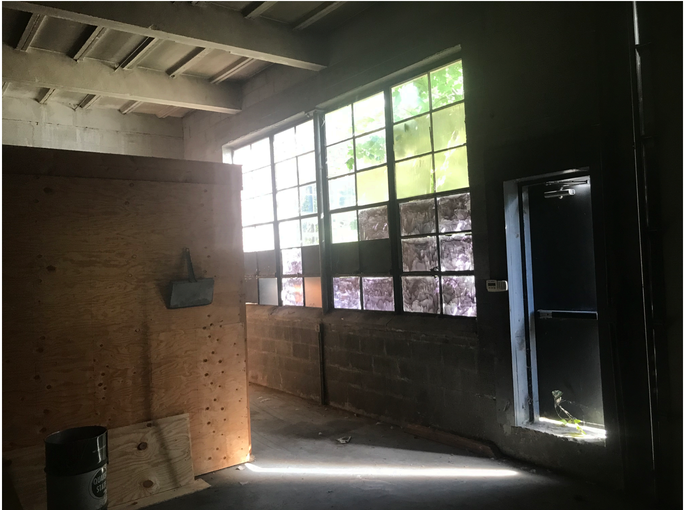
Photograph – 3: Photo depicts the typical condition and installation of asbestos and presumed asbestos window materials thermal the structure located at 32-60 Ernest Street; Providence, RI.
