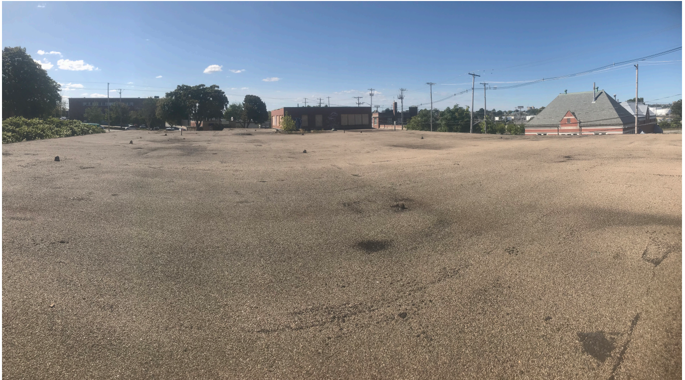
Photograph – 5: Photo depicts the typical condition of the roof area located at 32-60 Ernest Street; Providence, RI.
