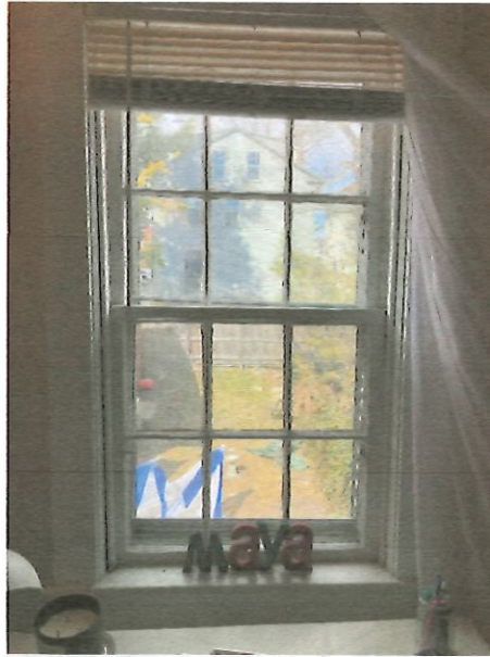
7 - 6/6 to be replaced
