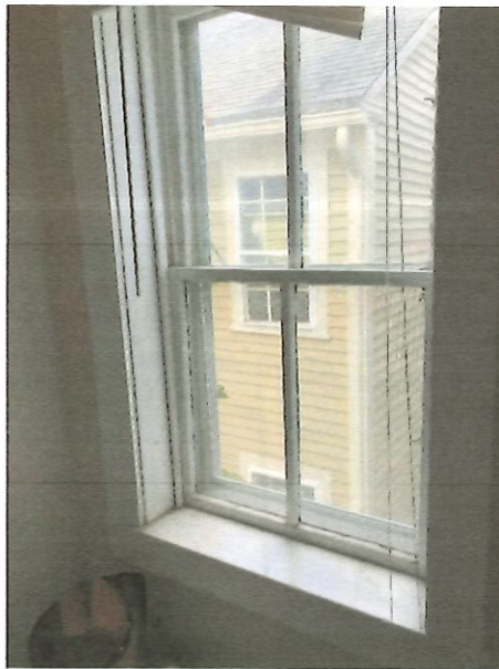
8 2/2 to be replaced
