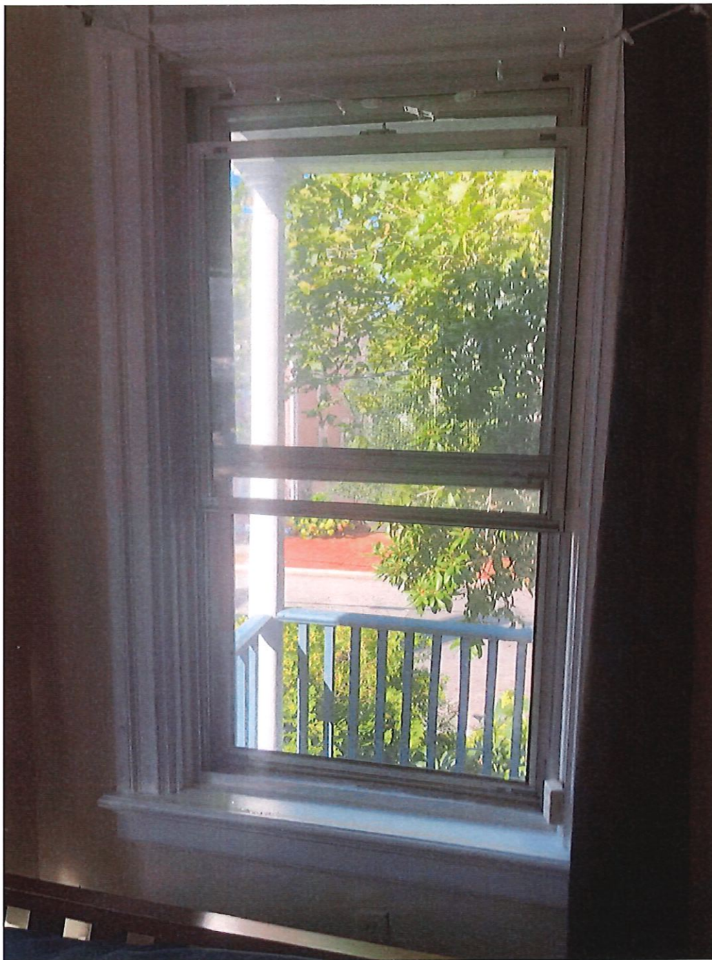
8 - Aluminum window from interior
