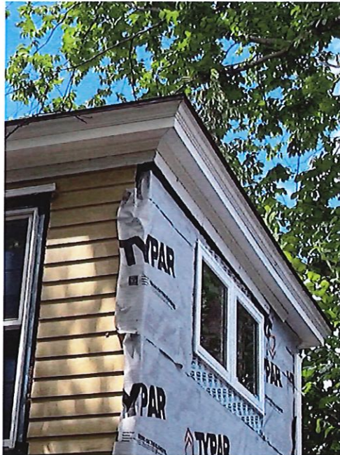
Figure 8 - New unit "M"
