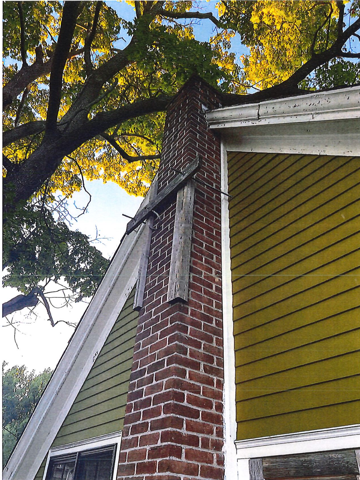
Photo: Chimney Unstable
