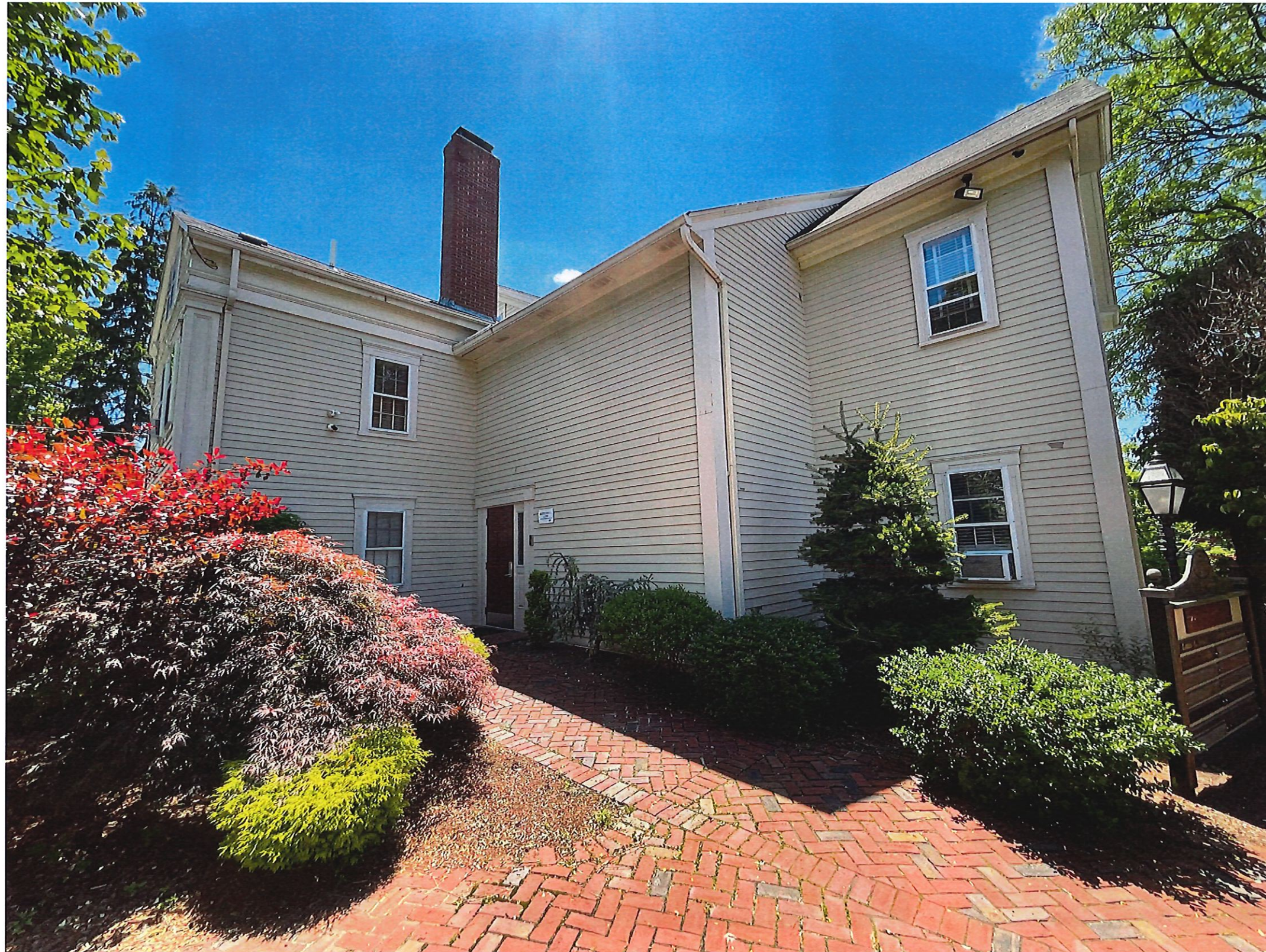
EXISTING NORTH EAST CORNER OF BUILDING AT LOCATION OF PROPOSED EXTERIOR STAIRCASE
