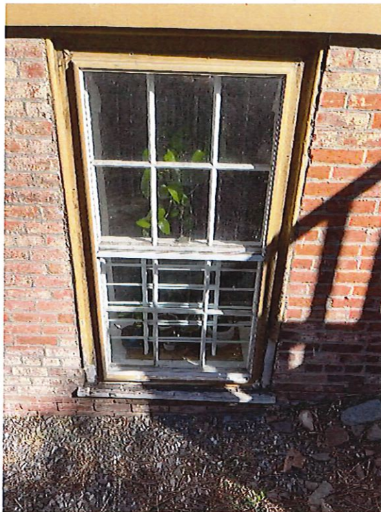
Figure 7 – Unit "A" at basement
