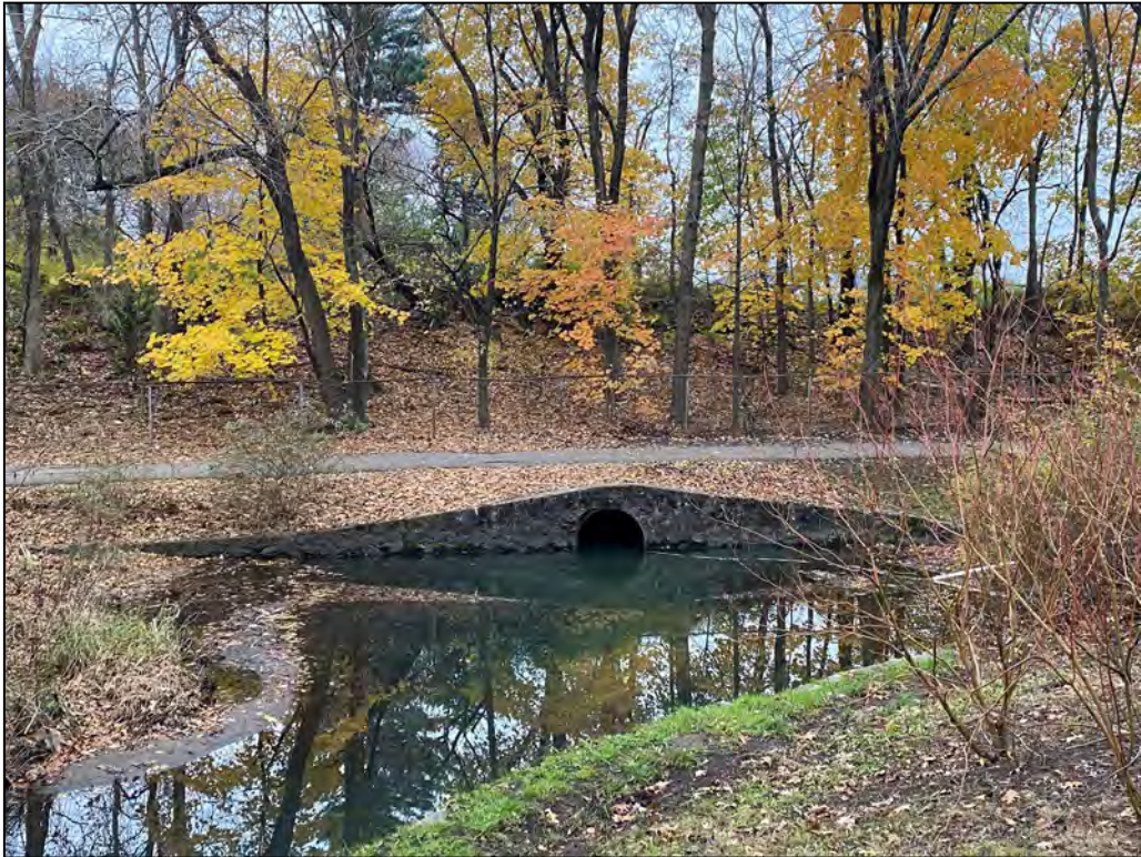
Photo No. 4: View of the 48-inch pipe outlet that discharges flow from Mashapaug Pond to Roosevelt Lake.
