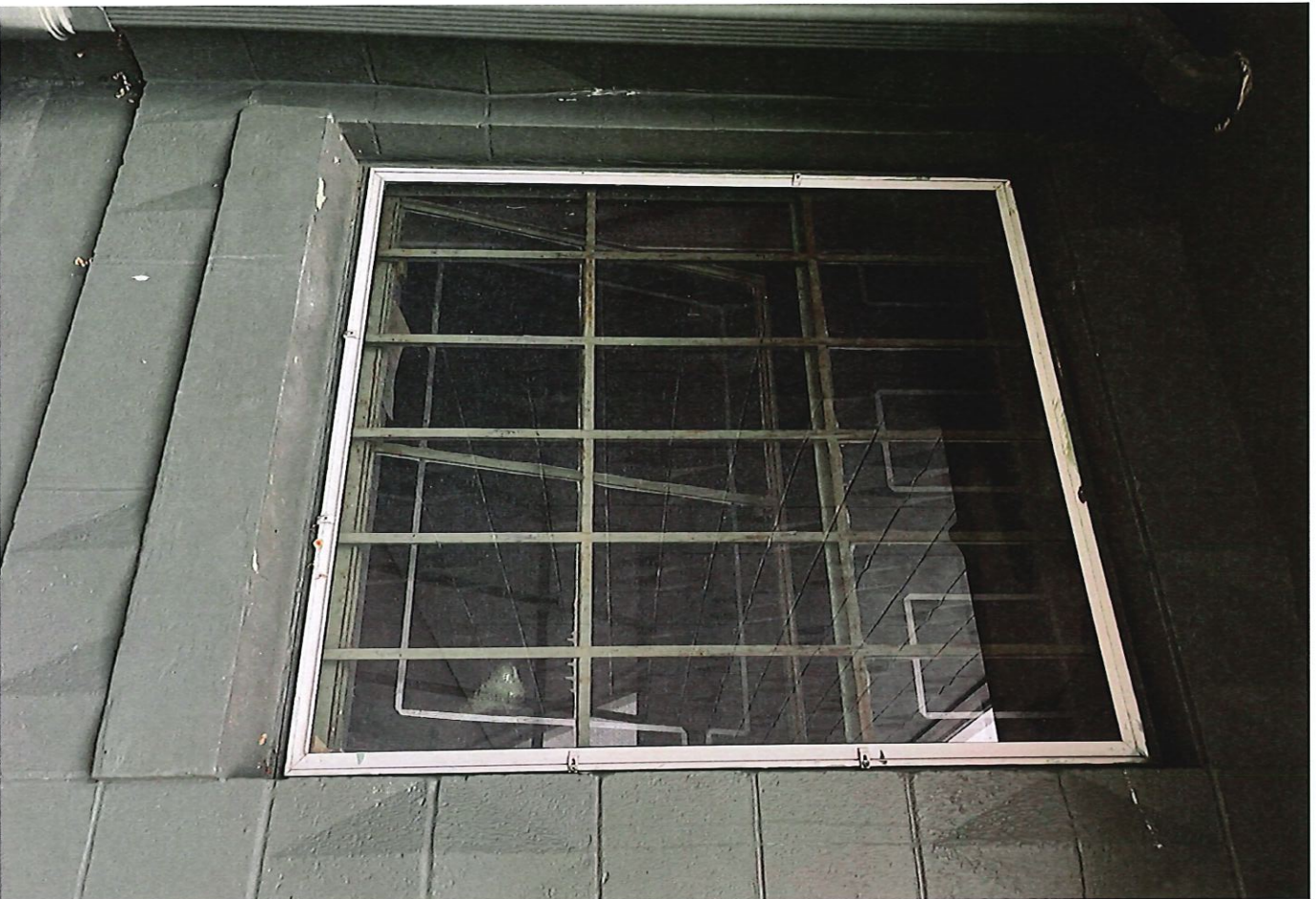
Front Window (For Replacement)
