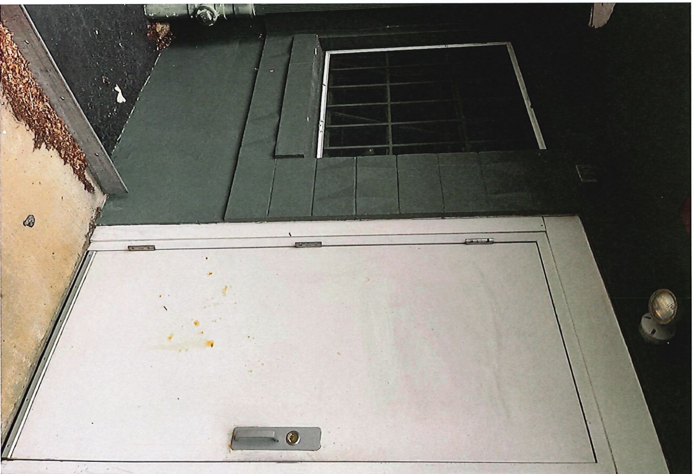
Front Door (For Replacement)
