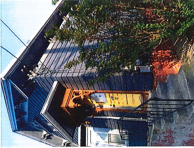
Existing Electric Service Meter with New Solar PV Disconnect
