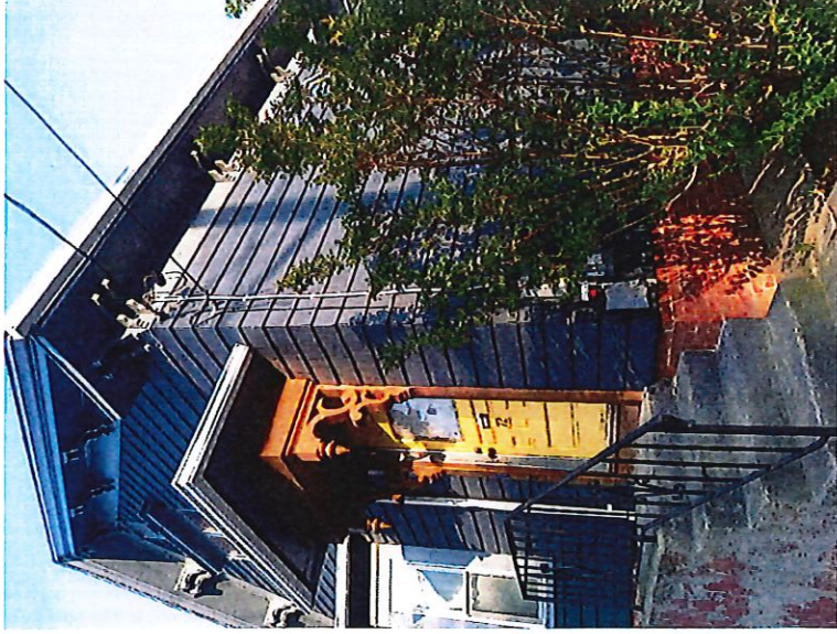
Existing Electric Service Meter with New Solar PV Disconnect
