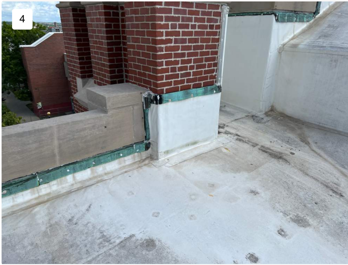
Anomaly - wet insulation - marked with spray paint
