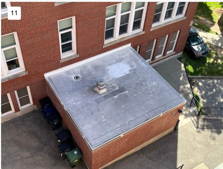
Anomaly - wet insulation - marked with spray paint
