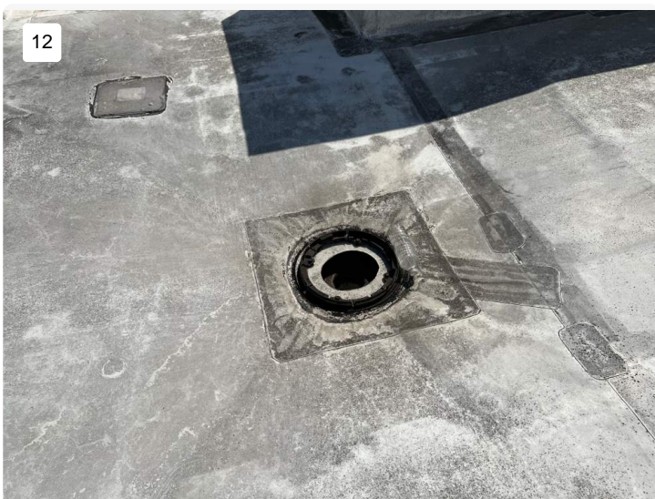
Missing drain strainer
