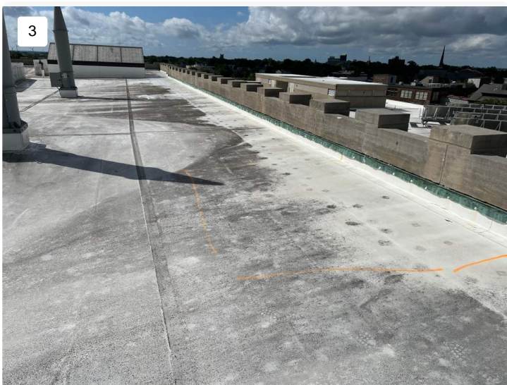
Anomaly - wet insulation - marked with spray paint
