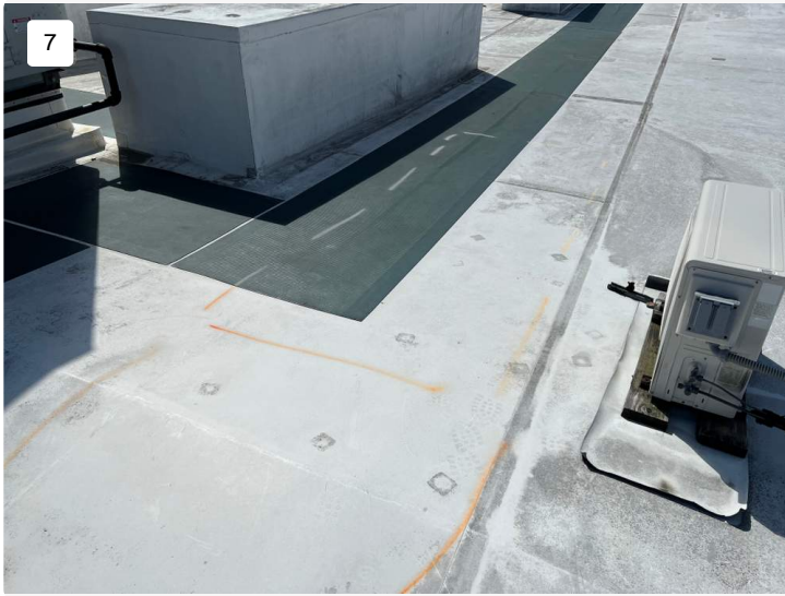
Anomaly - wet insulation - marked with spray paint
