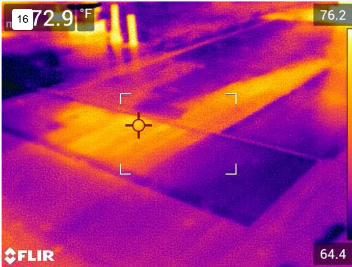
Thermogram identifying anomaly (wet insulation) in the roof assembly.
