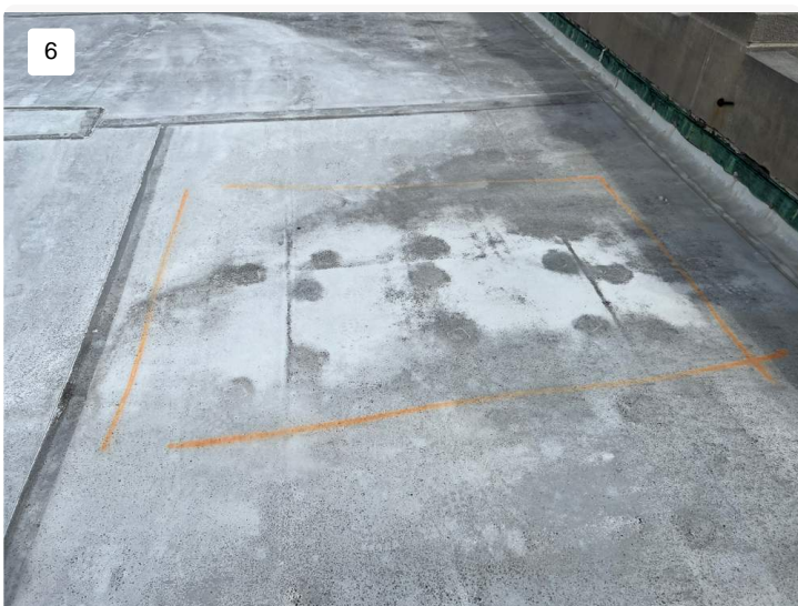
Anomaly - wet insulation - marked with spray paint
