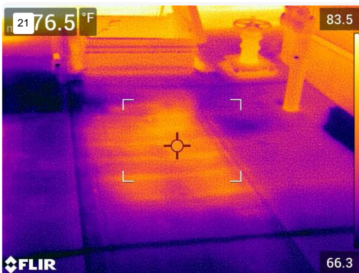
Thermogram identifying anomaly (wet insulation) in the roof assembly.
