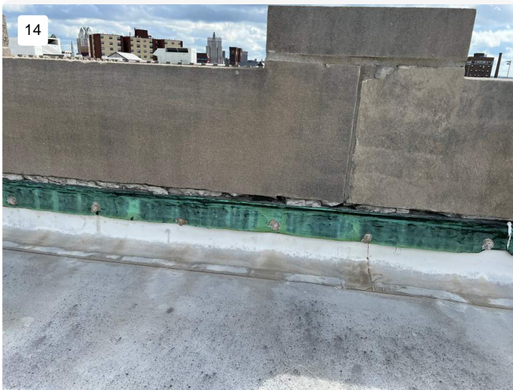
Deteriorated mortar joint at copper thru-wall flashing - typical
