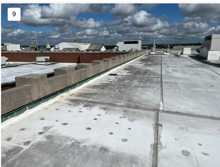
Anomaly - wet insulation - marked with spray paint
