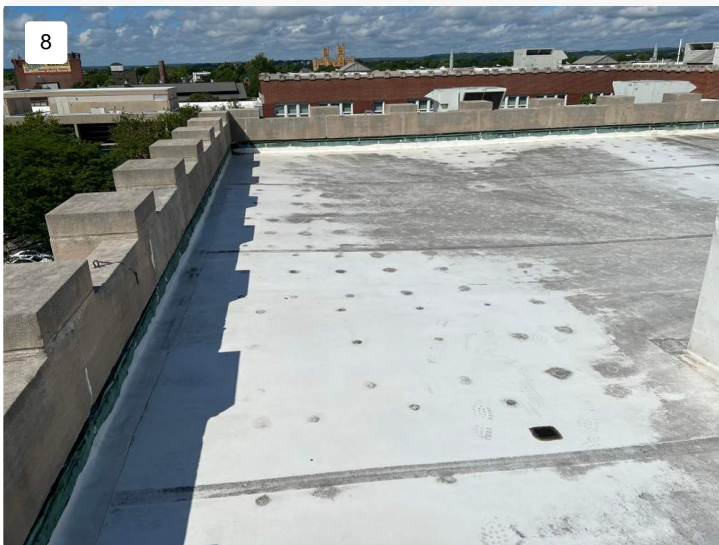
Anomaly - wet insulation - marked with spray paint
