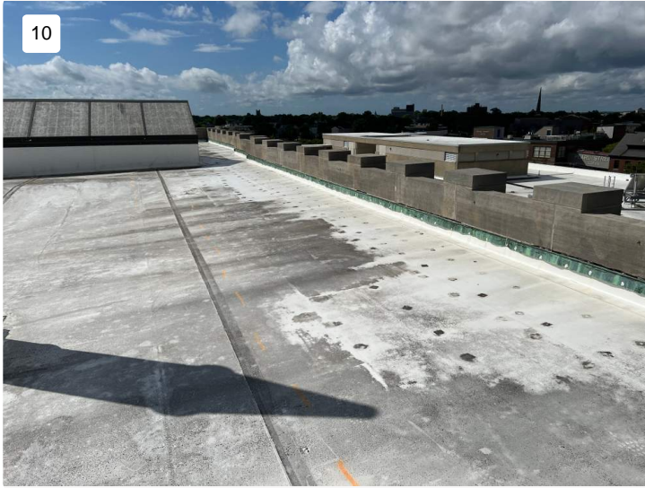
Anomaly - wet insulation - marked with spray paint
