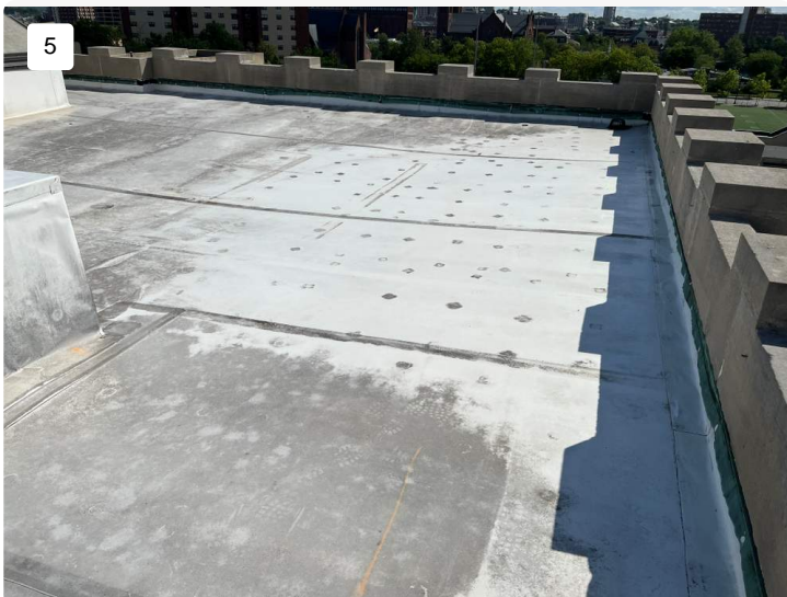
Anomaly - wet insulation - marked with spray paint
