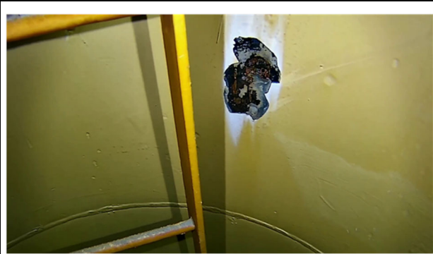
30) 6:47-Delamination inside riser pipe
