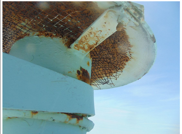
17) 17-Corrosion on vent and damaged screen
