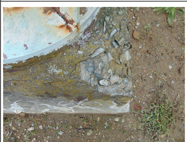
5) 5-Spalling on concrete foundation pad
