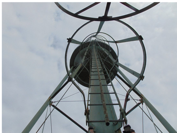
9) 9-Ladder with safety cage
