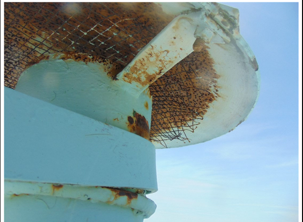
17) 17-Corrosion on vent and damaged screen
