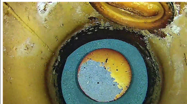
31) 8:18-Bottom of riser pipe with inlet/outlet
