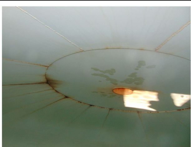
19) 19-Corrosion on interior weld seams
