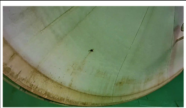
22) 1:51-Corrosion cell on roof
