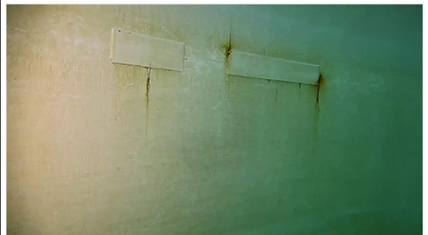
24) 3:15-Corrosion around patch plates
