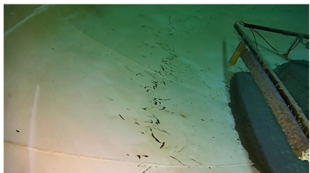
27) 5:14-Intact coating on bowl
