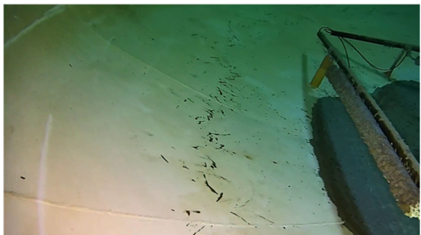
27) 5:14-Intact coating on bowl
