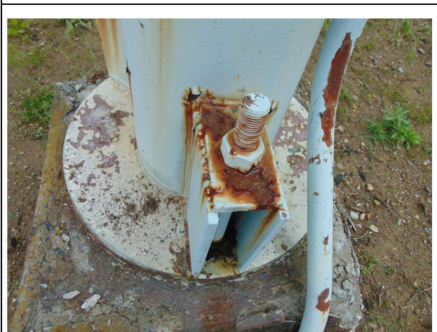
6) 6-Corrosion on anchor chair
