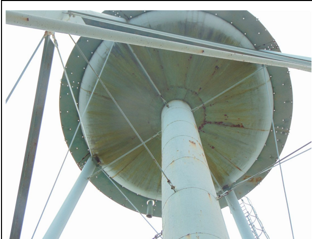
7) 7-Bottom of bowl with corrosion
