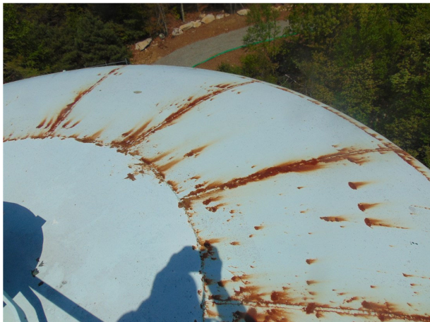
14) 14-Corrosion and delamination on the roof
