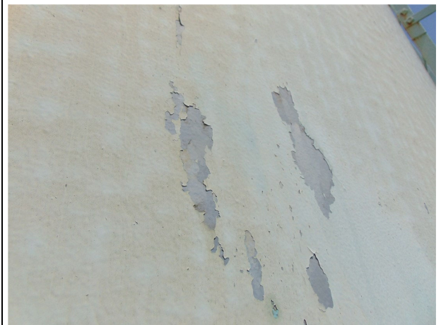
11) 11-Delamination on shell
