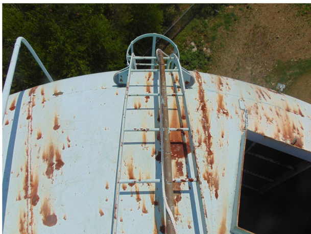
15) 15-Rotating roof ladder
