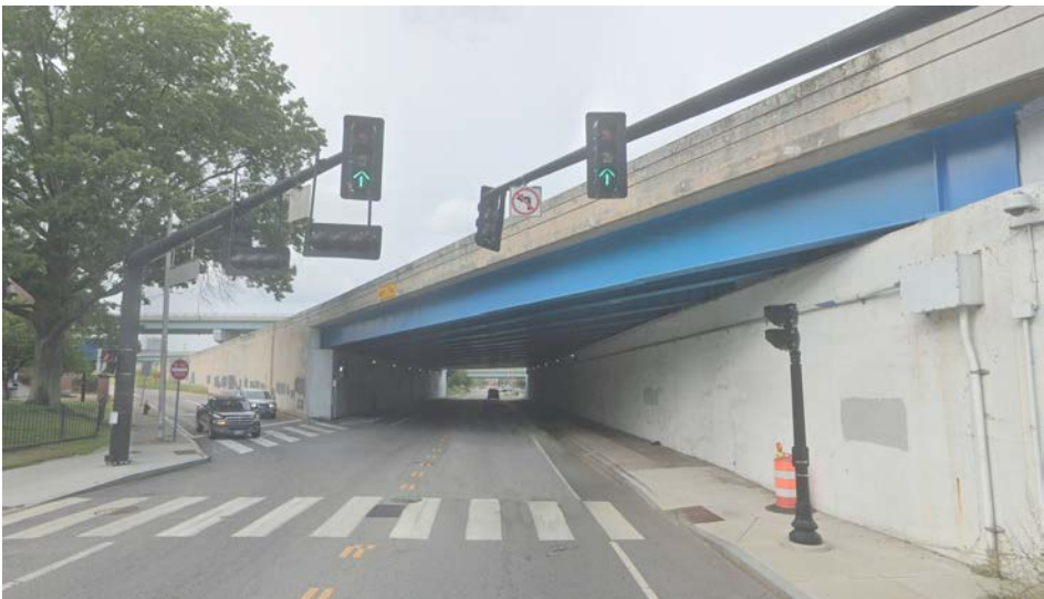
Eddy Street Underpass, current condition
