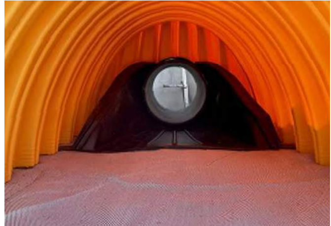
Looking down the Isolator Row PLUS
