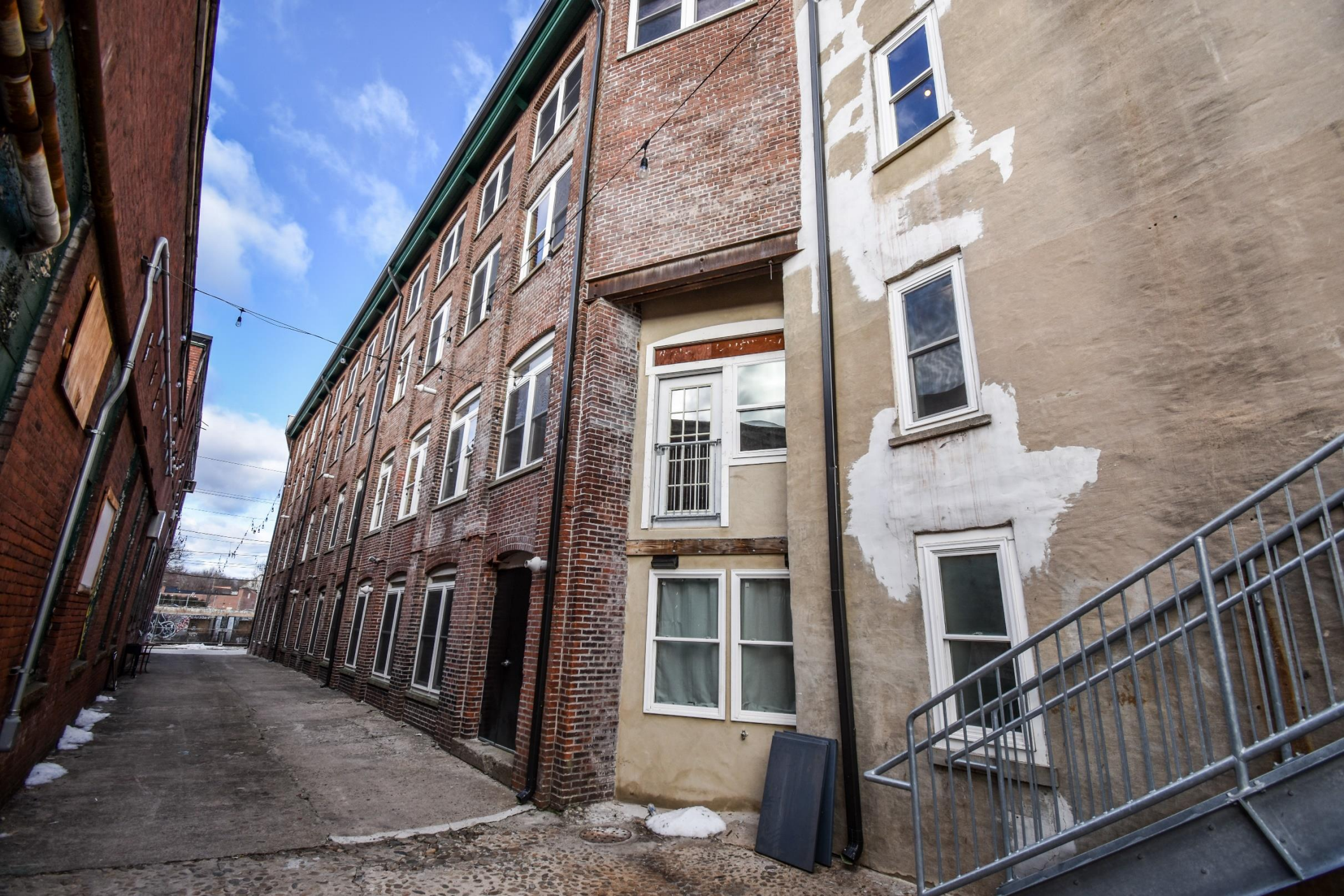
Photo 5. (L-R) (40 Agnes Street at far left) Addition 2, Main Mill from south alley, view west
