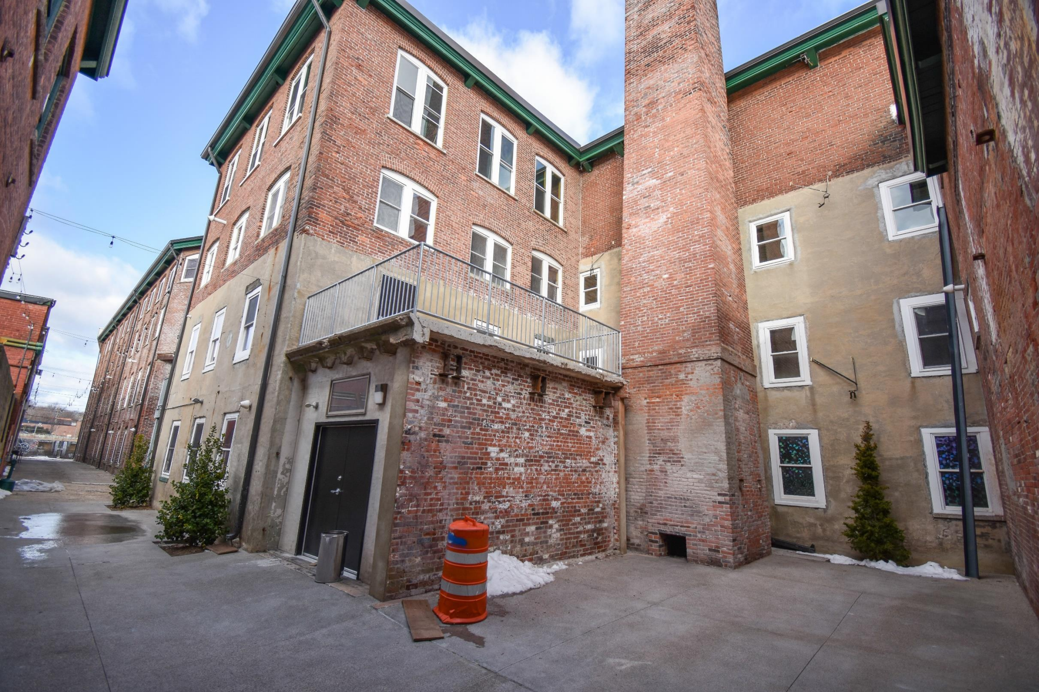
Photo 2. (L-R) Addition 2, First Engine/Boiler House with cotton storage/other extension in foreground Chimney, Main Mill, Addition 1 at south alley, view northwest
