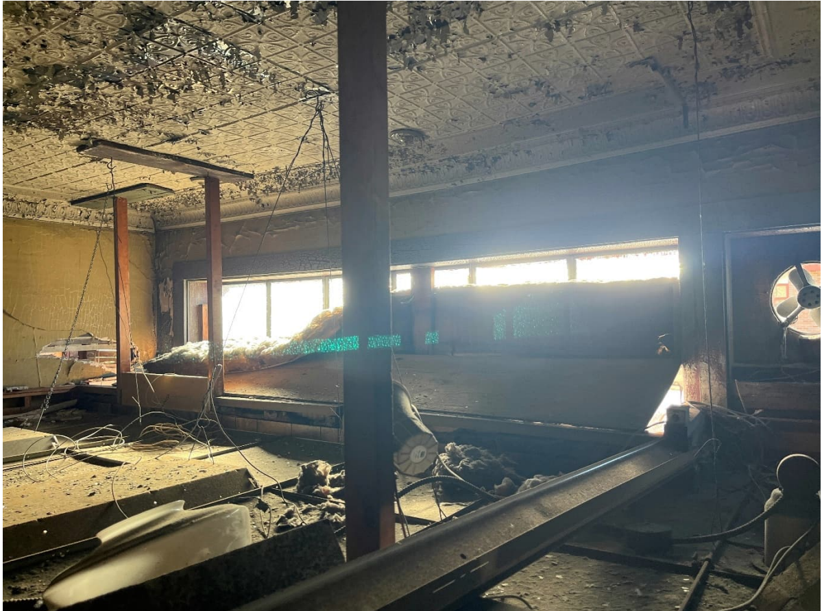
Photo 13 – Southern Portion, first story western half looking southeast. View from above the existing drop ceiling. Note the deflection in the header beam above the western storefront window. The observed second story floor/wall separation is directly above this location.
