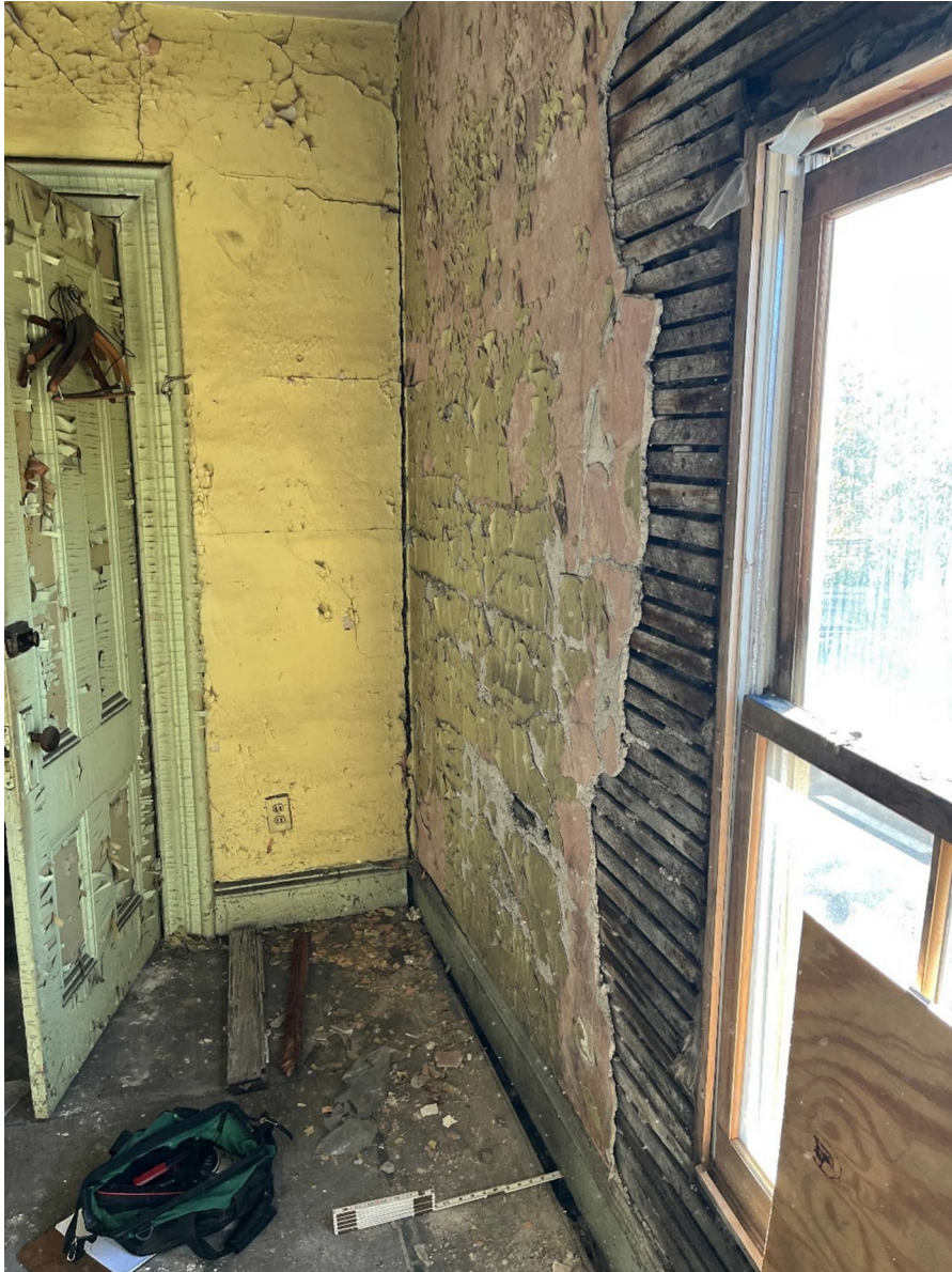
Photo 20 – Southern Portion, second story southwest chamber looking east. Note the ~1¾" separation of the floor and wall planes extends upward through the intersecting wall. The wall gap is wider at the base than at the top, indicating an outward movement caused by rotting floor framing and deflection of the underlying storefront window header beam.
