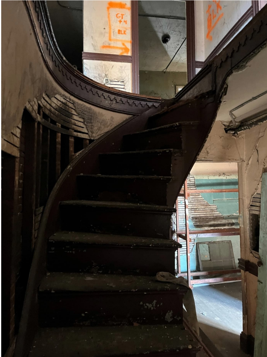
Photo 21 – Southern Portion, second story looking north. The once elegant curved staircase leads to the third story. Note damages due to neglect, vandalism, and active water infiltration from the failed roof membrane. The staircase sags discernably to the inside of the curve.
