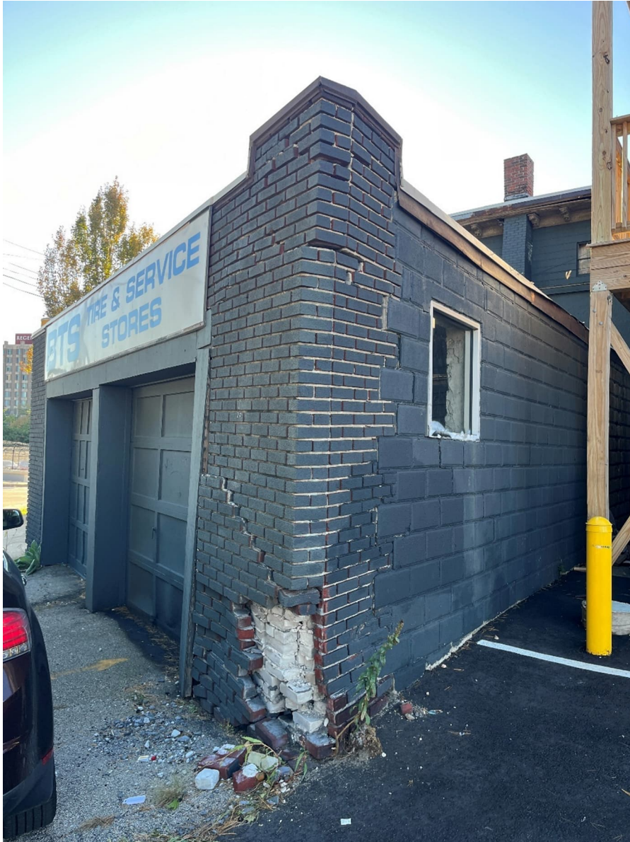
Photo 10 - 113 Broadway, Northern portion looking Southeast. Note extensive vehicular impact damage to the northwest corner of the building.
