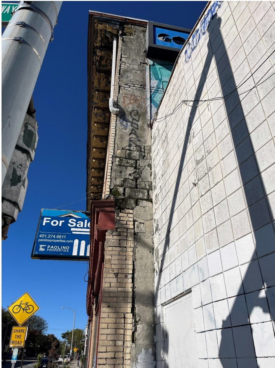
Photo 7 – 113 Broadway Southeast corner of building looking West. Note the separation of the brick veneer from the wood substrate is clearly visible in the form of a 1"± wide crack over the entire building height. Also note the lack of a decorative soffit overhang at the East wall of the "southeast protrusion".
