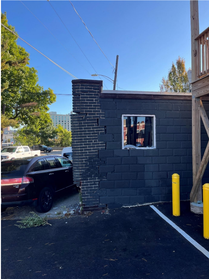
Photo 11 - 113 Broadway, Northern portion looking East. Note extensive vehicular impact damage to the northwest corner of the building. While visually impressive, the lesser damaged western CMU wall is load bearing, not the heavily damaged northern brick wall.
