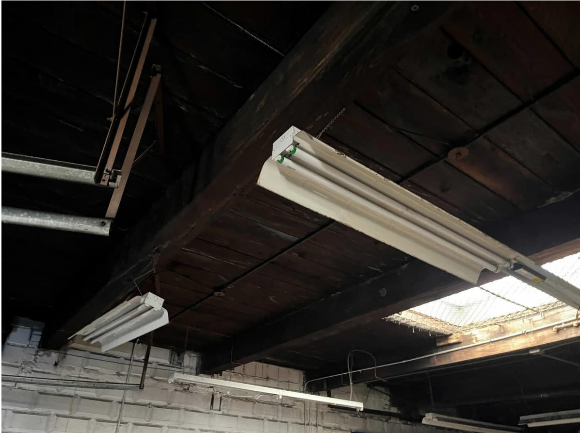
Photo 24 – Northern Portion, typical interior view looking east. Note the typical construction – CMU block walls with heavy wood timber rafters. Some water damage and active infiltration was noted but overall the roof structure appeared to be intact.
