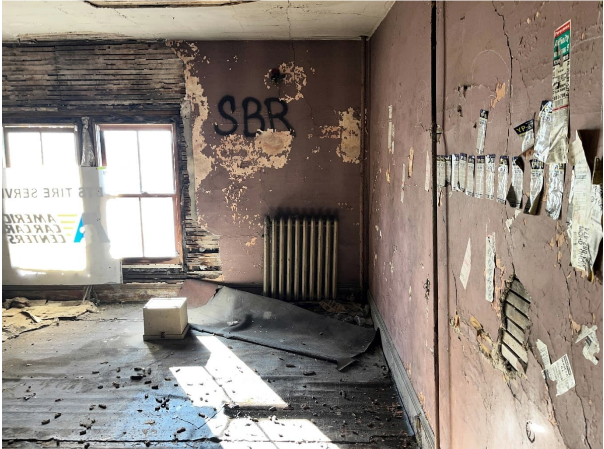
Photo 17 – Southern Portion, second story southeast chamber looking south. This is the “southeast protrusion”. Note the crooked radiator which indicates the out of level floor. Also note the wall, ceiling, and floor damages due to active water infiltration through the failed roof membrane.
