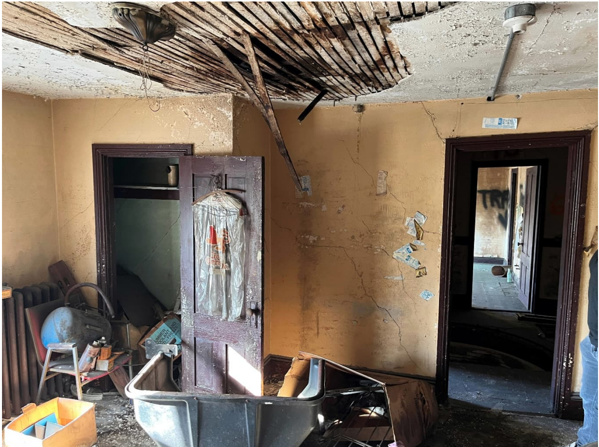
Photo 22 – Southern Portion, third story southeast chamber looking west. This is the “southeast protrusion”. Note the severely sloped floor as indicated by the crooked doorway trim and diagonal shear cracking on the walls. Also note the ceiling damages due to active water infiltration through the failed roof membrane.
