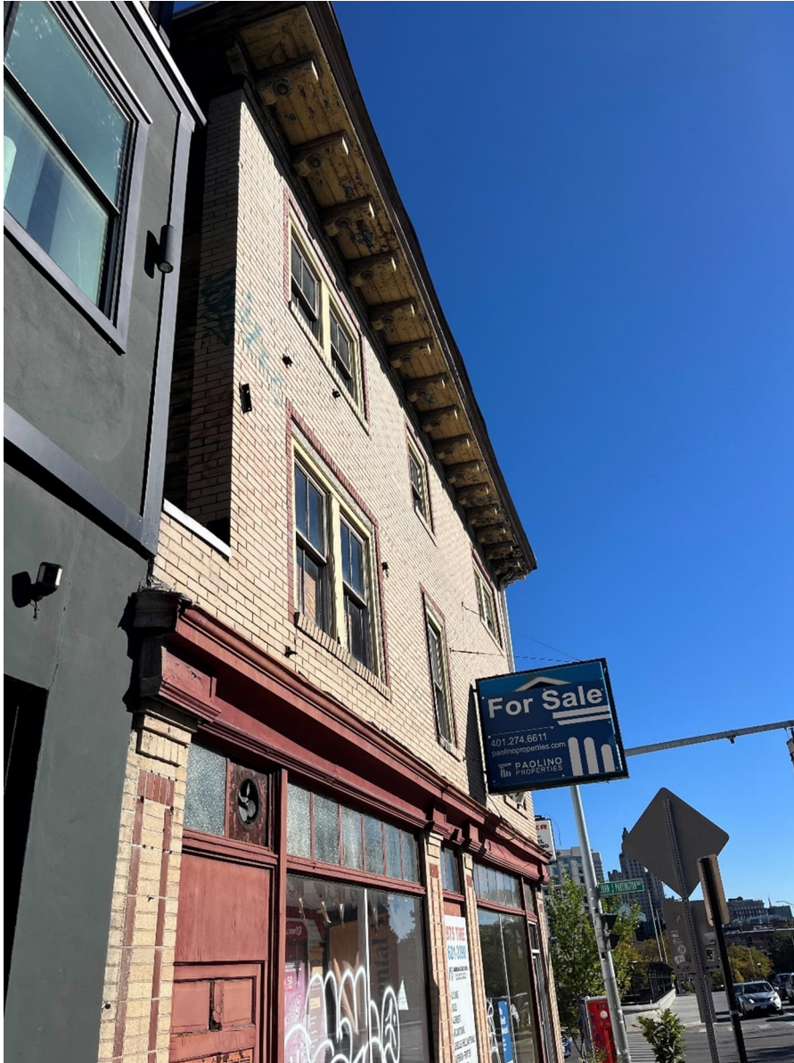
Photo 6 – 113 Broadway South Elevation looking Northeast. Note undulations of building façade caused by a combination of structurally inadequate framing and the separation of the brick veneer from the wood substrate.
