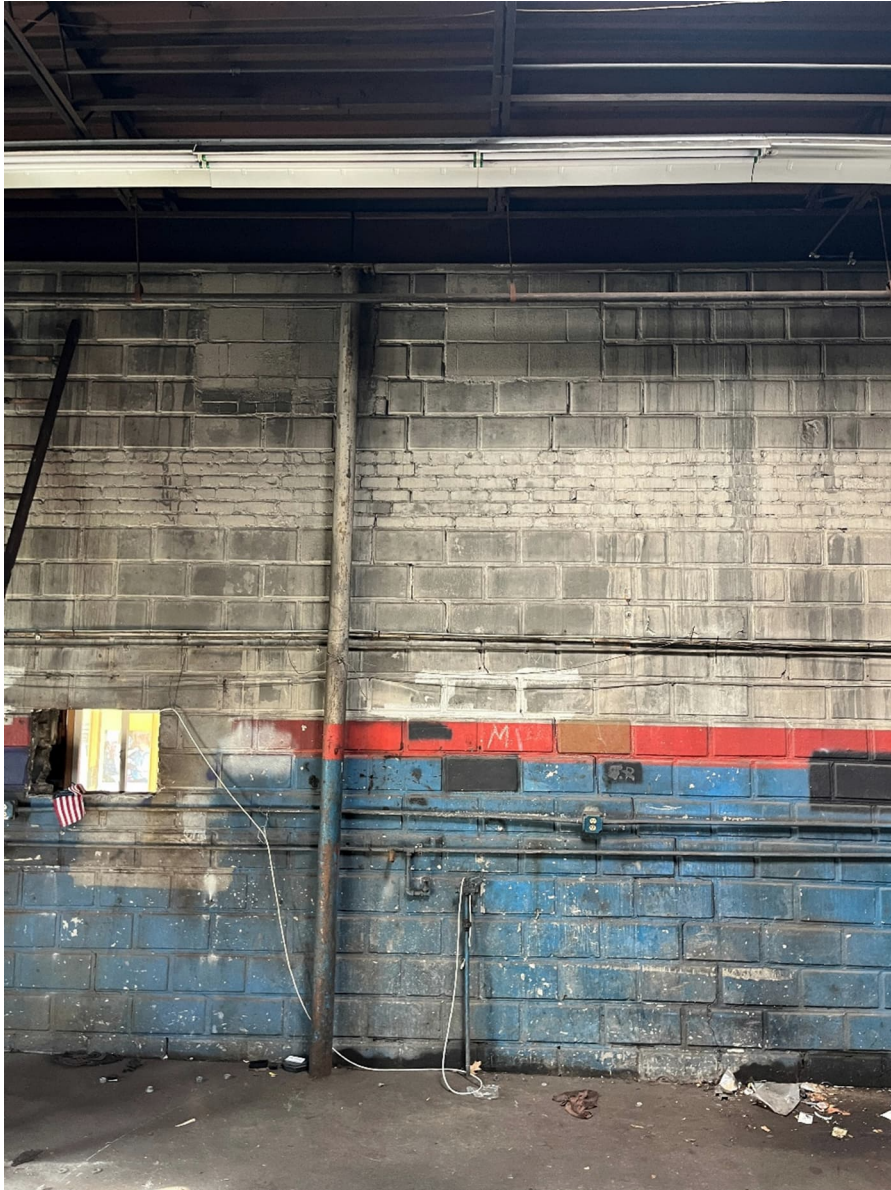
Photo 26 – Eastern Portion, typical interior view looking west. View of the steel header beam and steel columns which support the west ends of the open web steel joists. Note the step cracking in the “southeast protrusion” CMU wall, indicating foundation distress.
