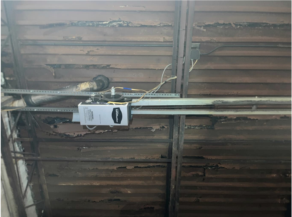
Photo 28 – Eastern Portion, looking west/up. Detail of severely water damaged corrugated metal roof panels. Active water infiltration through the roof was not noted at the time of our inspection, presumably due to the installation of another layer of roofing material above.
