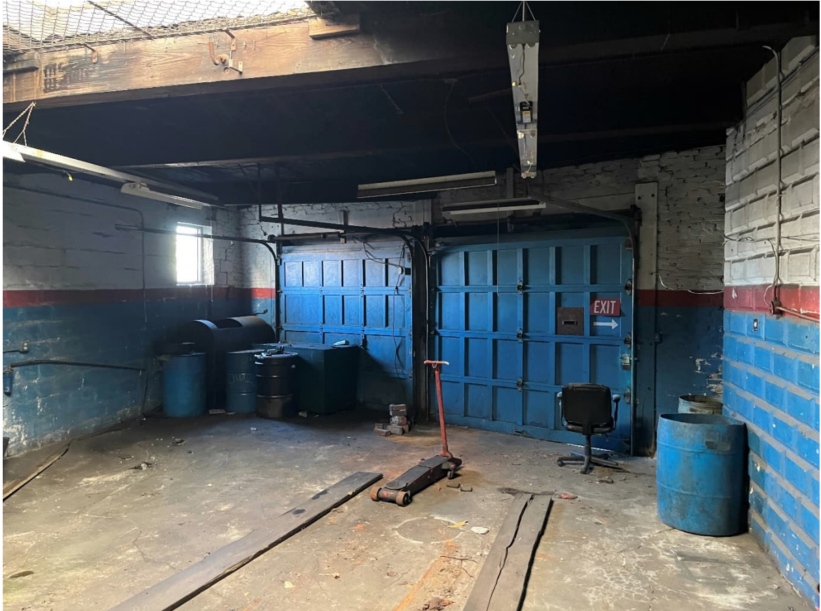
Photo 23 – Northern Portion, typical interior view looking north. The vehicle-damaged wall is located in the background left corner. Note the typical construction – CMU block walls with heavy wood timber rafters.
