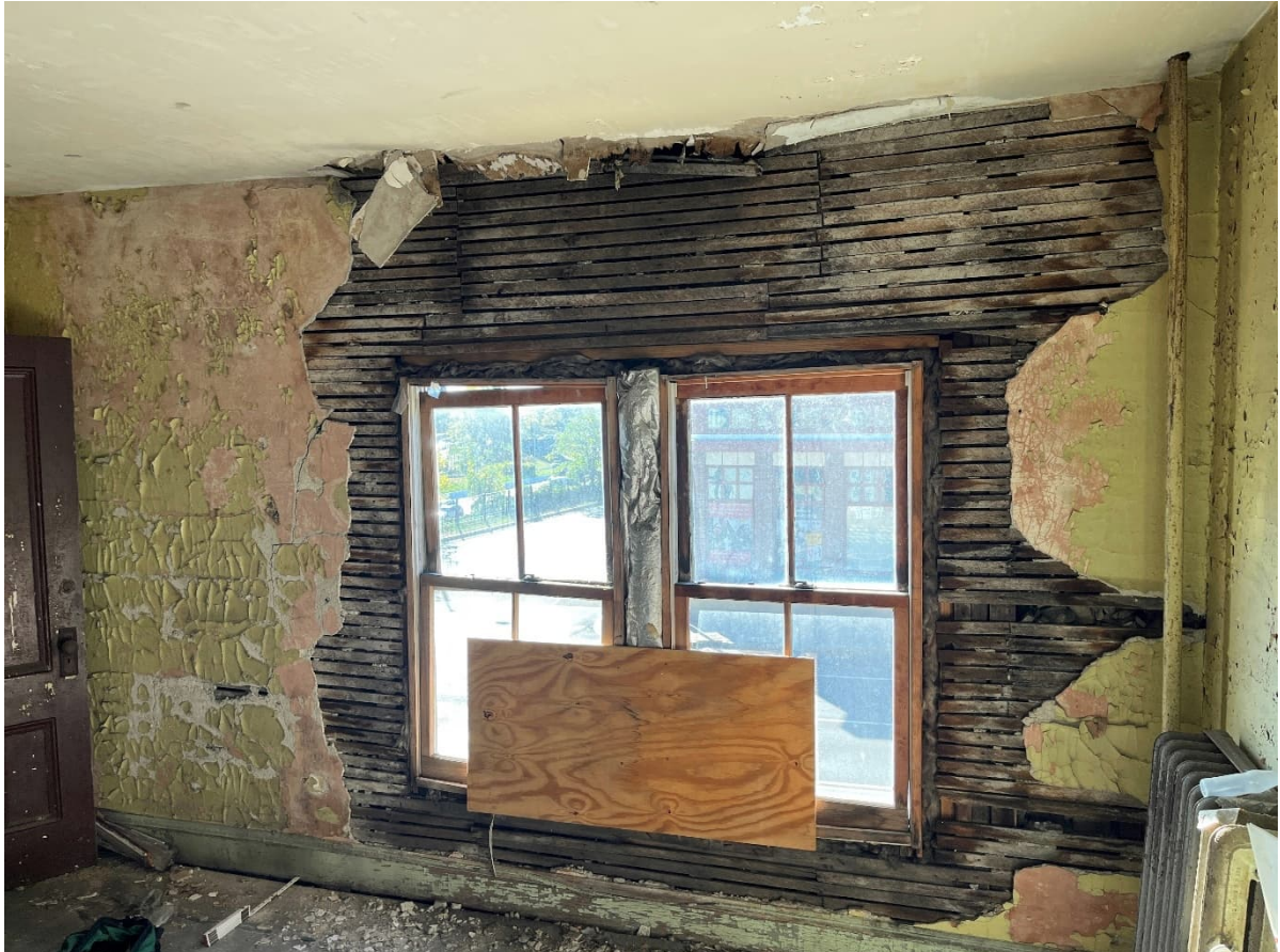
Photo 18 – Southern Portion, second story southwest chamber looking south. Note the wall, ceiling, and floor damages due to active water infiltration through the failed roof membrane. The wall is separated from the floor framing by ~1¾" (note measuring ruler on the floor).
