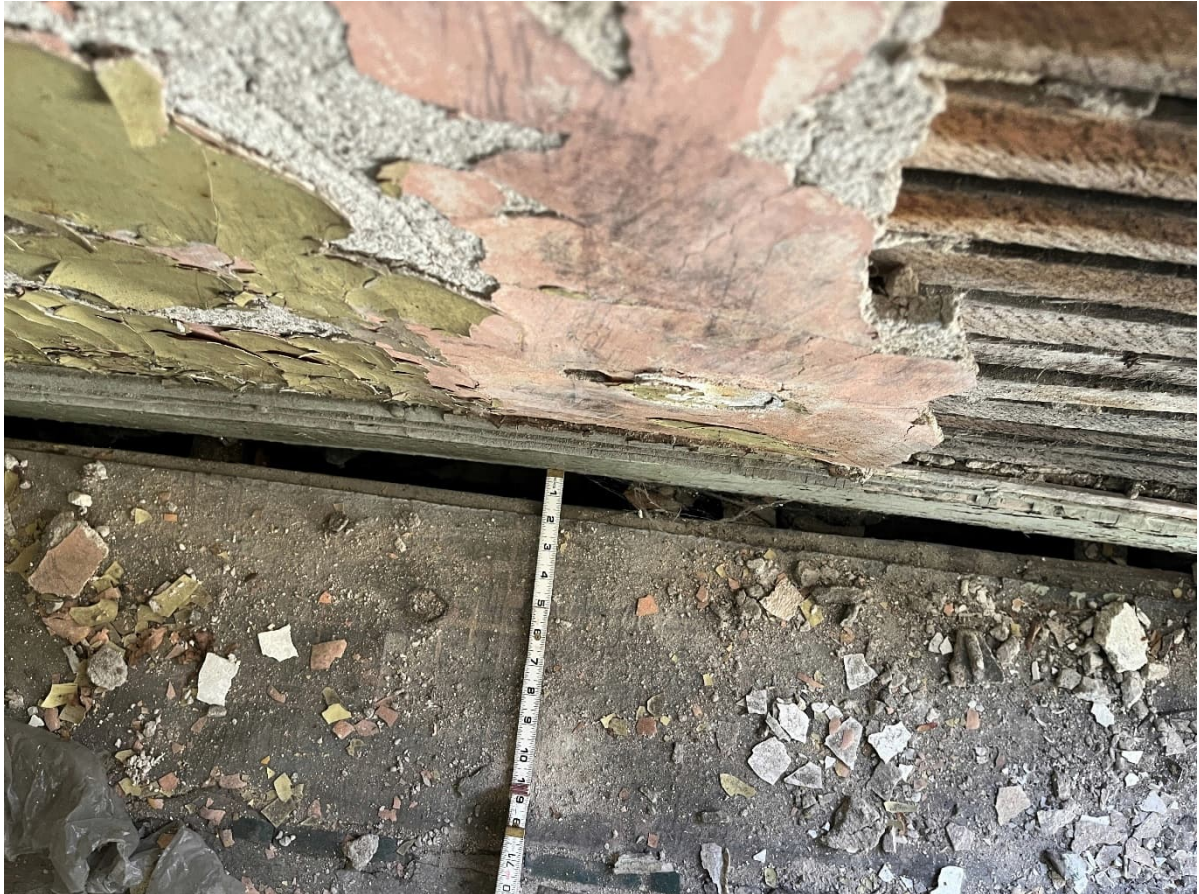
Photo 19 – Southern Portion, second story southwest chamber looking south/down. Detail of ~1¾" separation of floor and wall planes. Rotten floor joists were visible through this gap.
