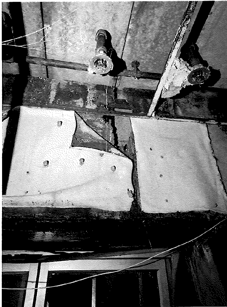
015: Image of fire protection heads
